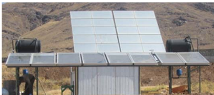
Fig. 6 Simultaneous testing of various types of solar collectors.
