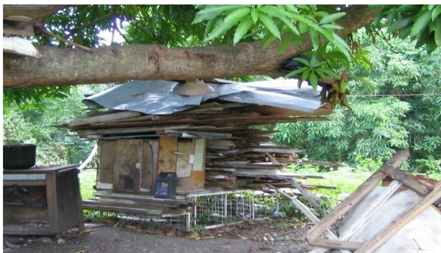
Figures 4 & 5: Dwellings at the entrance to the Parry Town informal settlement, and building materials from a dismantled house. Source: © Sheere Brooks.
