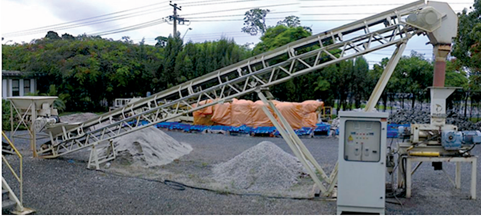
Figure 1 Pilot HPGR facility.
