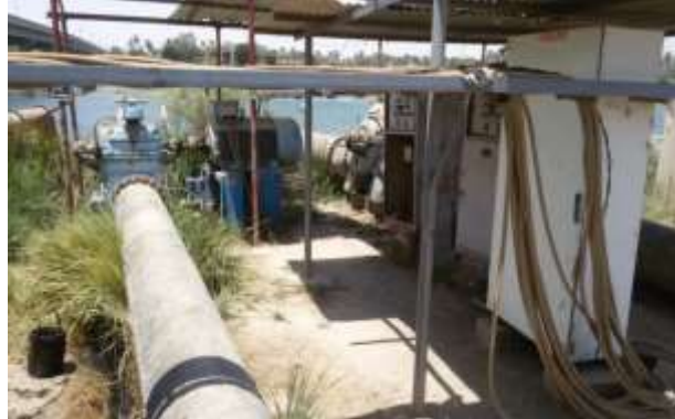
Figure (1). Pumps installed on the Euphrates River
