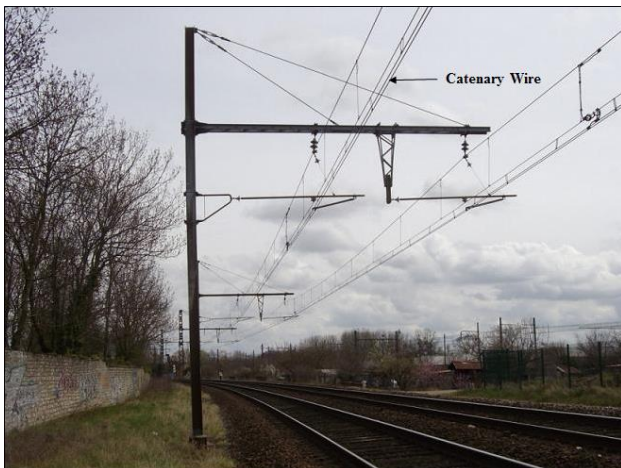
Figure 3: Example of the catenary using 1,500 V voltage.
