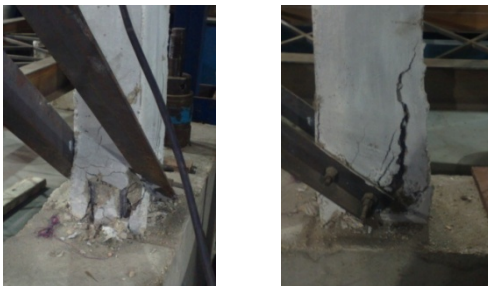
Figure 5. Mode of failure of F3
