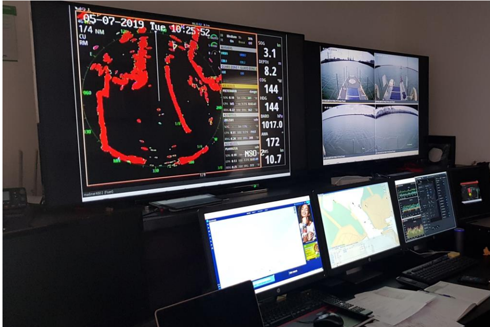
Figure 2. Shore Mission Control Station providing access to K-MATE Autonomy Controller and Situational Awareness System (photo: K. Zwolak).
