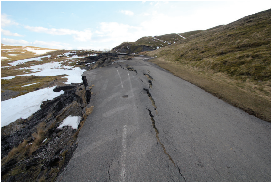
Fig. 1.5. Damage to the A625 carriageway by the Mam Tor landslide, Derbyshire (photo credit: David Giles).
