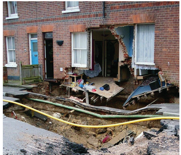
Fig. 1.15. Major subsidence through chalk mine crown hole collapse, Field Road, Reading, Berkshire (photo credit: Clive Edmonds).
